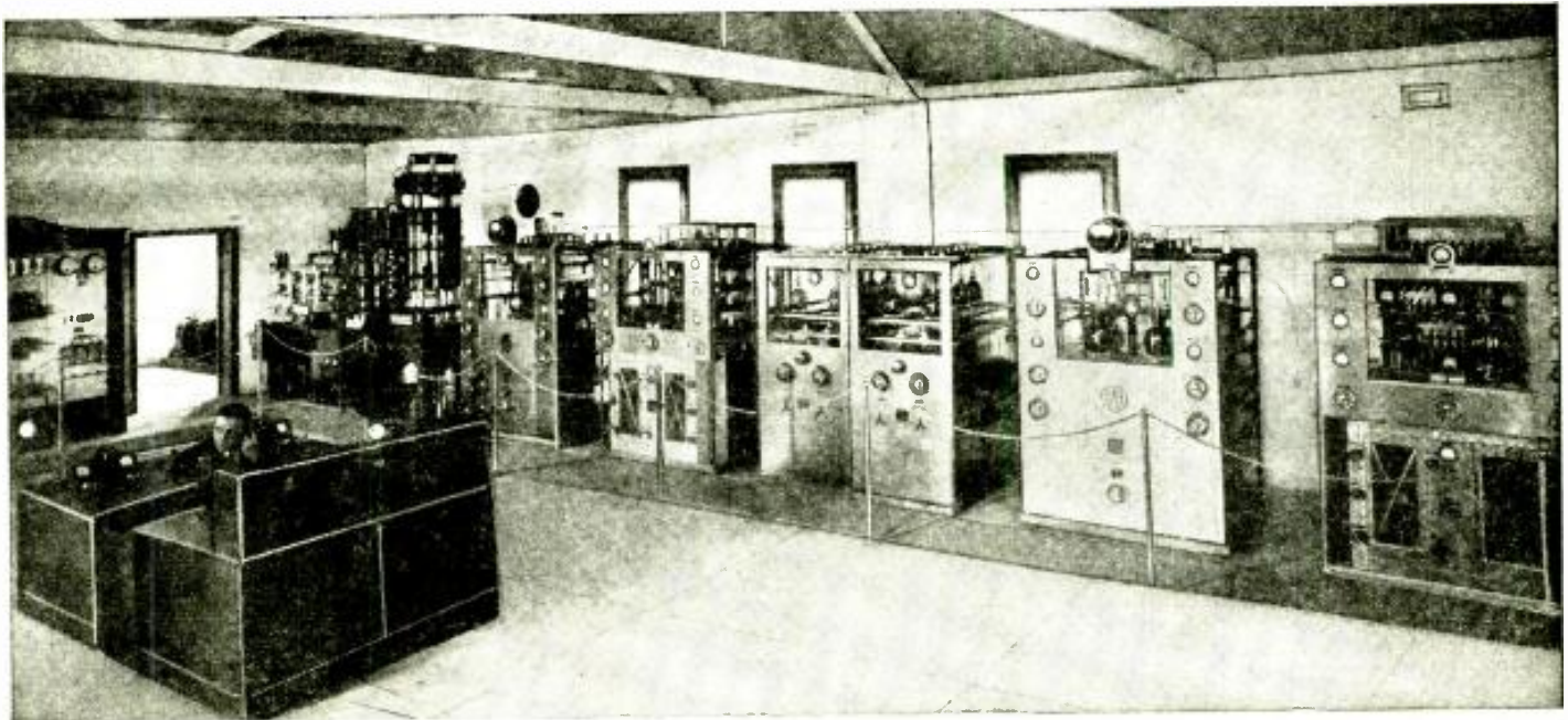
The transmitter of station VK3ME, Melbourne, situated at Radio Centre, Braybrook, Victoria. This Australian-designed and manufactured transmitter is used in the World-wide Broadcasting Services of VK3ME.
